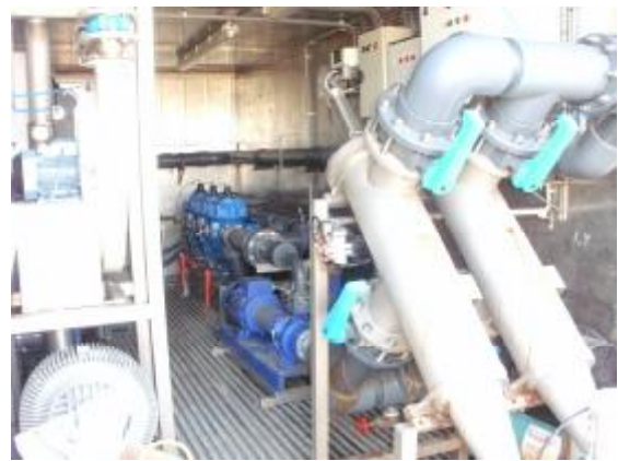
Filterset in de filtercontainer
