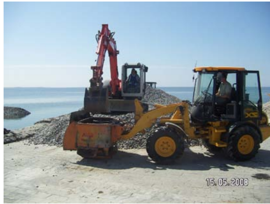
The crushed rocks are filled in the compulsory mixer
