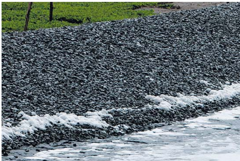
Figure 2-2: Exemplary photo of an Elastocoast revetment on the Hallig Langeness (Photo BASF PU)
