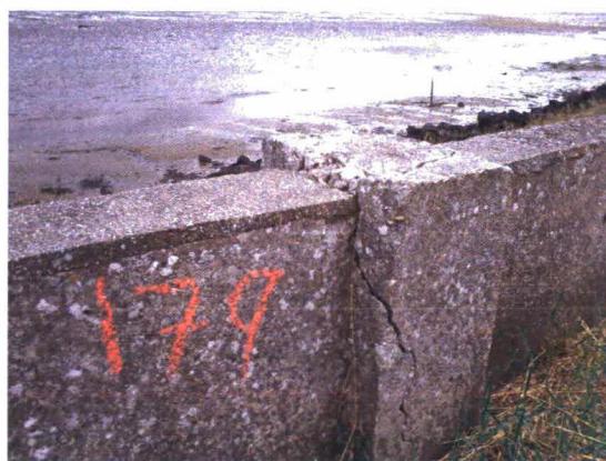
Plate 4: Viane, Dijkpaal No. 329 + 36.85m: Cracking in post.
