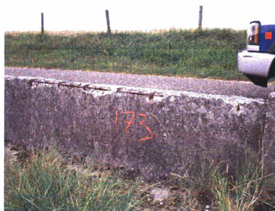
Plate 2: Viane, Dijkpaal No. 329 + c.55.5m: Reinforcement bars visible along top of wall.
